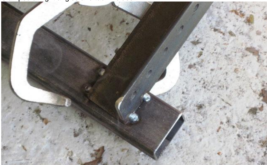
The parts successfully tack welded with the MIG welder. I had marked the position where the angle iron with holes in had to be welded to the box section with a ruler and a pair of odd leg callipers
