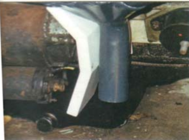
2-6-3-1 As you can see a block-hugger exhaust manifold passes very close to the starter motor and, consequently, some thermal protection is essential. I fabricated this steel shield and put fibreglass insulation inside it before ...
